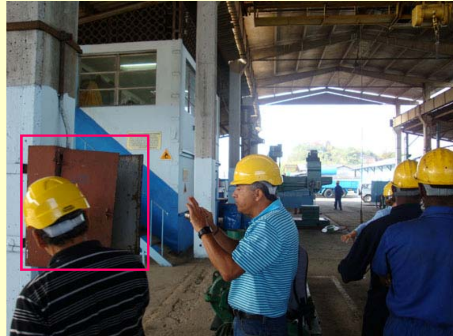
Defective main cabinet
