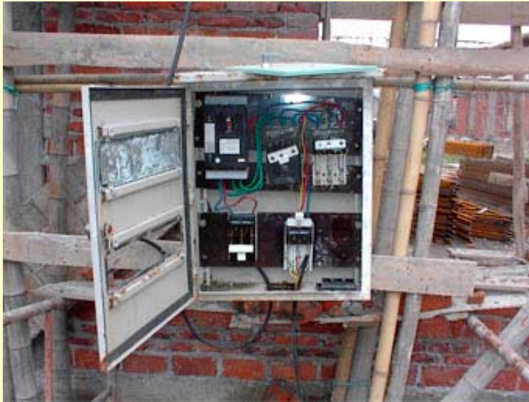
Defective construction site main cabinet
